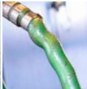
Old coupling with hose clamps causing leakage and pressure drop
